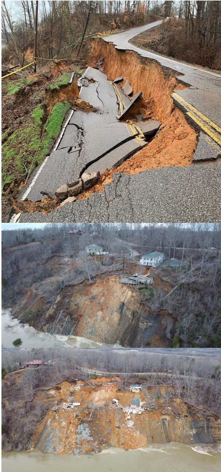
Mass wasting at Chalk Bluff in Hardin County, destroying two homes and a road. (photos via the Hardin County Fire Department)
