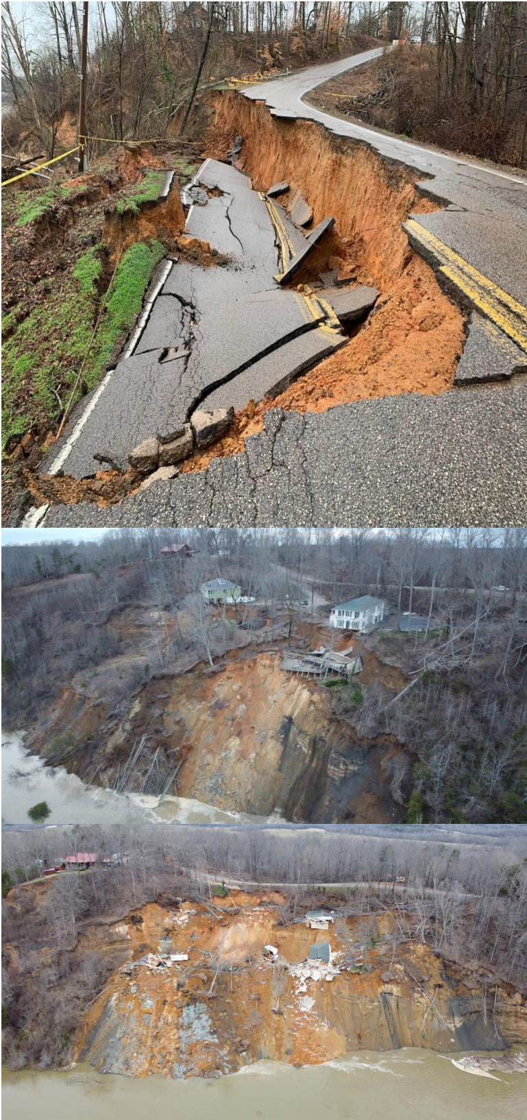
Mass wasting at Chalk Bluff in Hardin County, destroying two homes and a road (photos via the Hardin County Fire Department).
