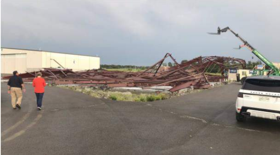
Damage to a hanger under construction at the Lebanon Municipal Airport in Wilson County. Image via News Channel 5 Nashville.
