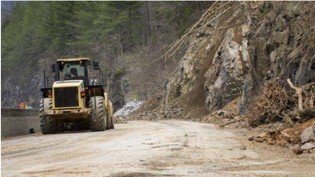
Rockslide that shut down I-40 just past the Tennessee-North Carolina State line. Photo via Citizen Times.
