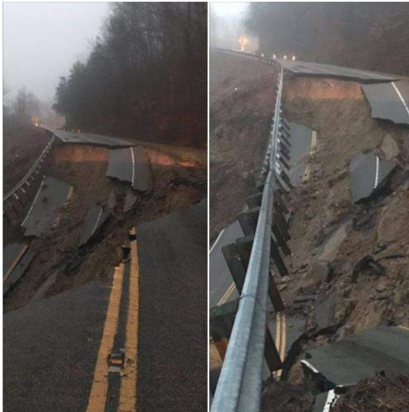
Damage to Hwy 70 in Hawkins County, due to a mudslide which occurred Feb 21 st and proved fatal. Photo via Mark Naigi (TDOT).
